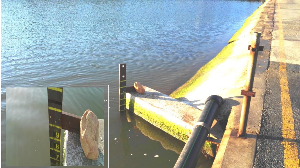
Figure 3 Extended buttress linked to the main culvert under the Seekoei Estuary. The top of the buttress is 100 mm below the roof of the culvert. The temporary gauge in the inset to this photograph shows that the water level is 300 mm below the top of the buttress (Photo: Billy Ives).
